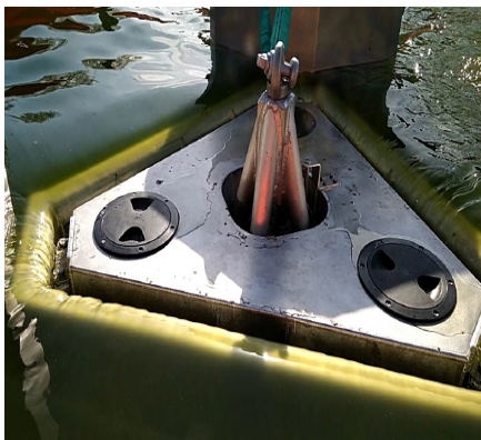
High capacity weir
